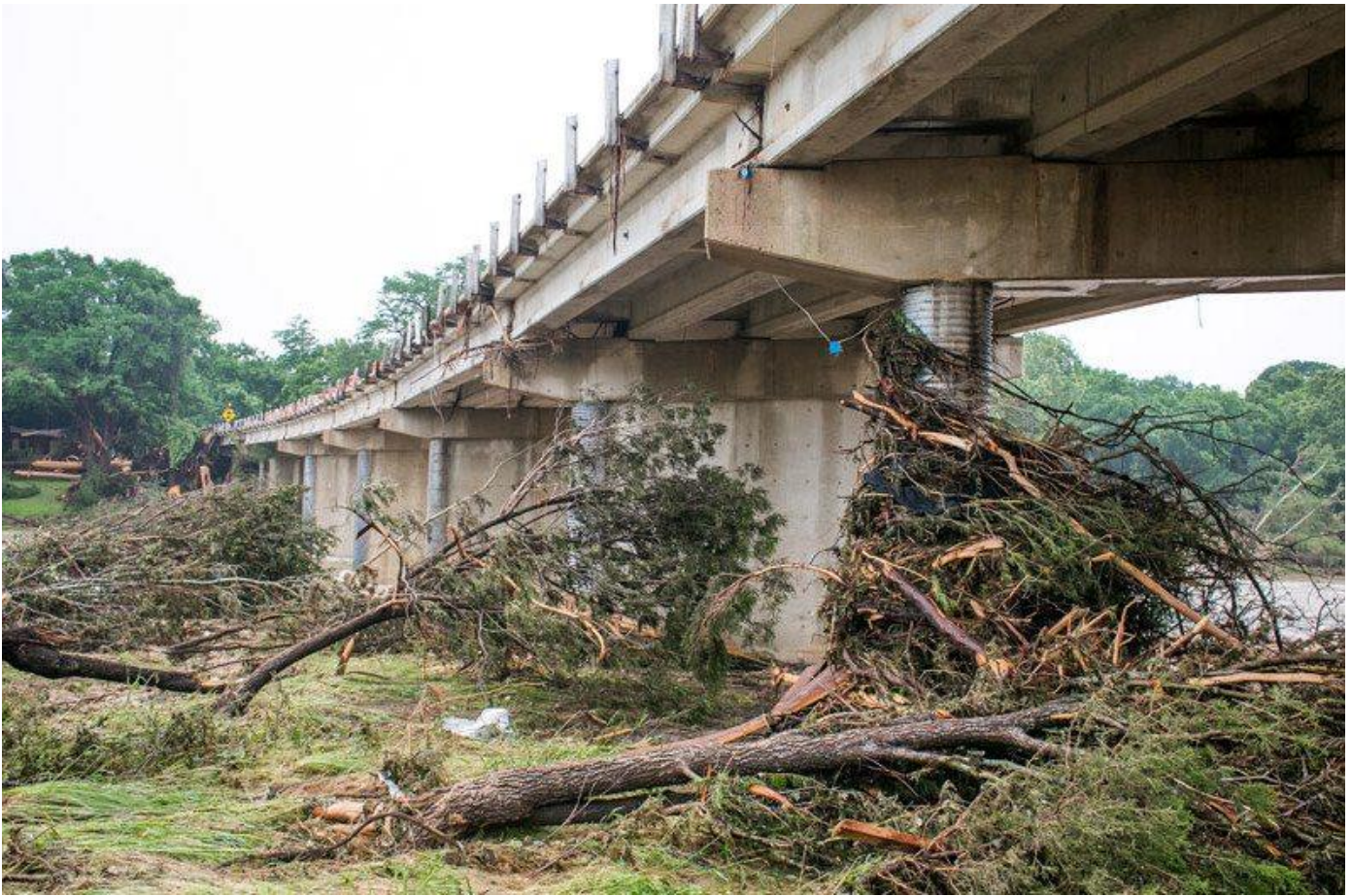
Figure 4: Damage Near the Blanco River Following the Memorial Day Flooding
